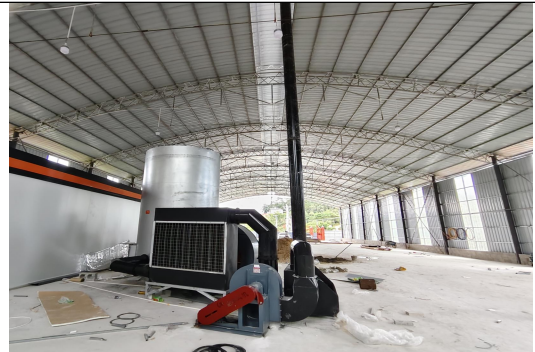
1#热风炉+1#水膜除尘器+DA001
